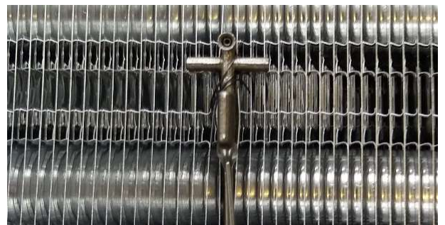
Figure 2 Probe (S_KPS_qxpj) mounted on radiator.
